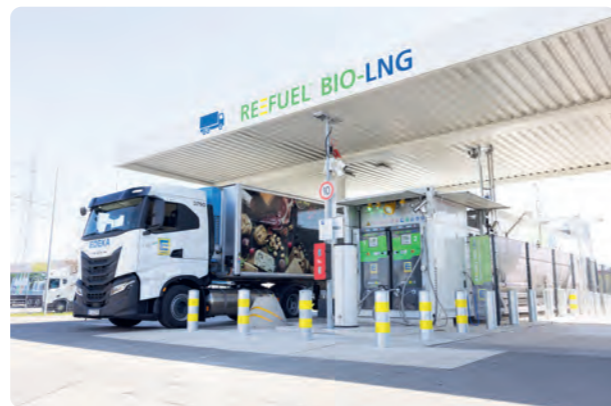
The eighth bio-LNG filling station within the EDEKA Group was put into operation at the beginning of this year in Freienbrink.
